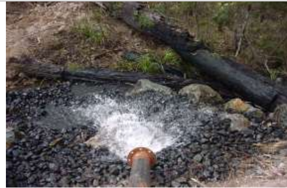
Figure: Treated waste water, now within the standards for drinking water, being discharged
